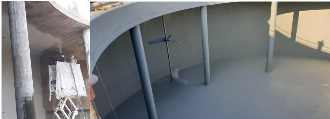
Photos: Application of Polyurea Rayston inside an anaerobic digester in a treatment plant in Italy (Lecce).
