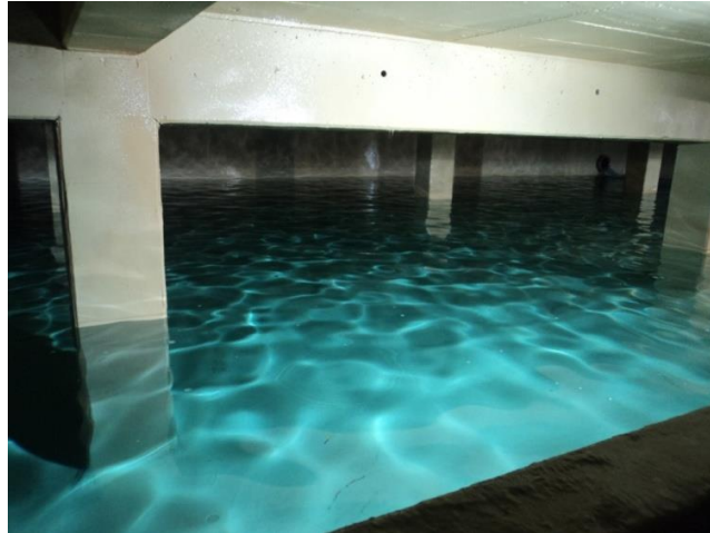
Photo: Process water tank, already in service, refurbished with Polyurea Rayston at the Seat automotive plant in Martorell (nearby Barcelona).
