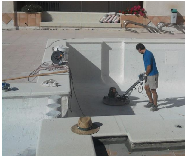
Photo: Treatment of a concrete surface with diamond grinding machine, as part of the preparation of the substrate, in a waterproofing process with Polyurea Rayston.
