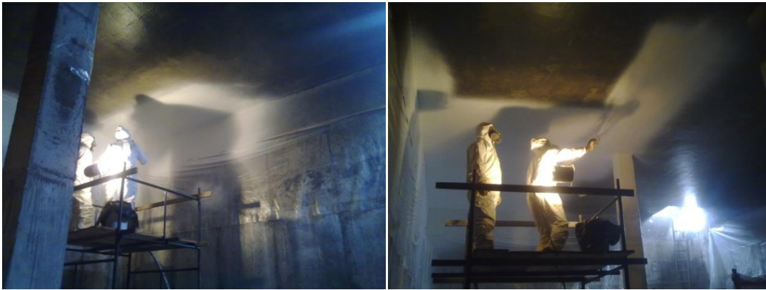
Photos: Application of Polyurea Rayston inside a tank at the WWTP of Itaperuçu - Sanepar (Brazil).
