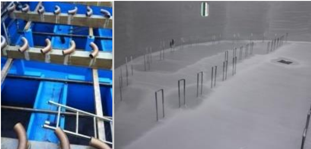
Photos: Final aspect of treatments with Polyurea Rayston. Digester in a WWTP in Seville and in a paper mill in Tortosa (Tarragona). Polyurea Rayston can be applied on supports other than concrete (metal, PVC pipes ...). In each case, a different primer compatible with each material must be applied.
