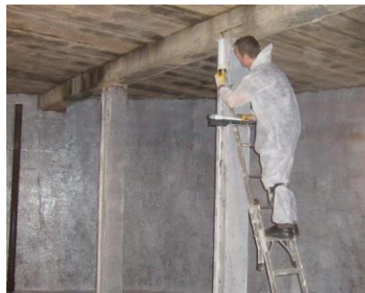
Photo: Application of Humidity Primer by roller in a drinking water tank in the town of Killone (Ireland). When applied, the resin has a whitish, milky appearance, which loses (becomes transparent) when it cures and the water it contains evaporates completely.
