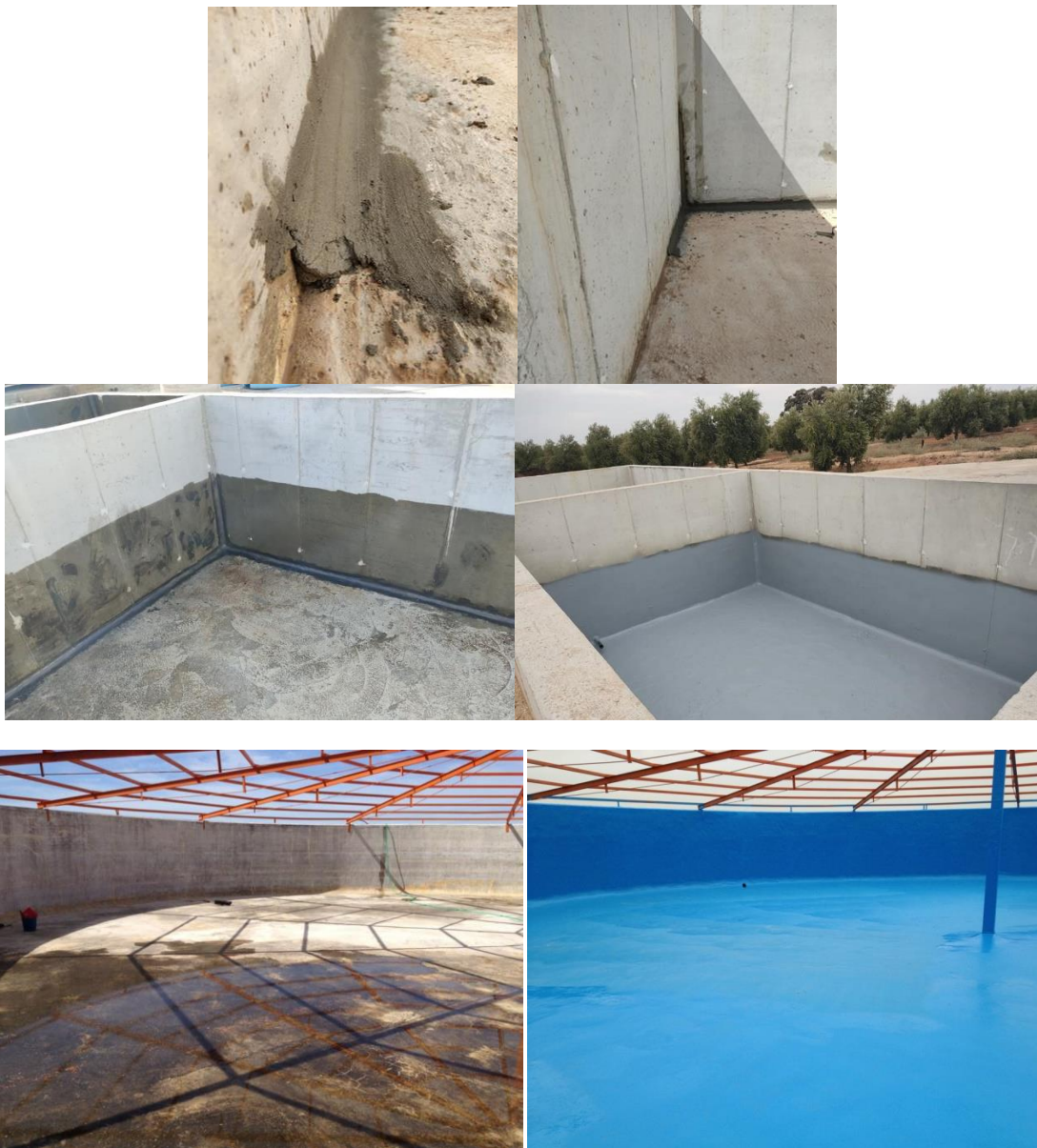
Photos: Water tanks in Andalusia, south of Spain, refurbished with Polyurea Rayston. The right angles were rounded before the application of the system, as described in this document.
