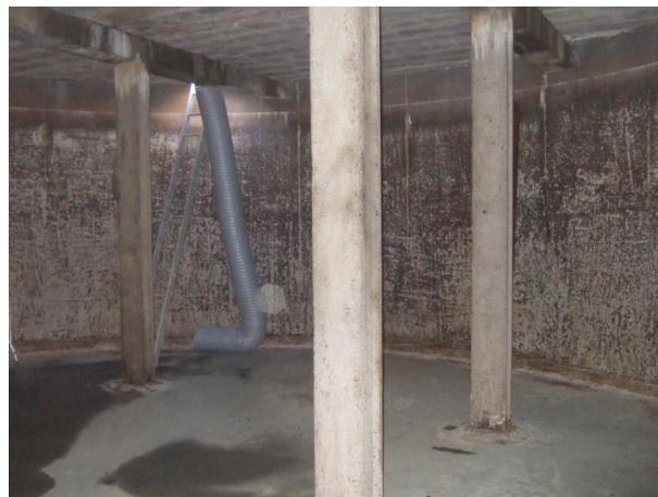
Photo: Forced ventilation in a drinking water tank in the town of Killone (Ireland) with the aim of drying completely the concrete surface, before proceeding with the application of the primer, after having properly prepared beforehand the said surface.
